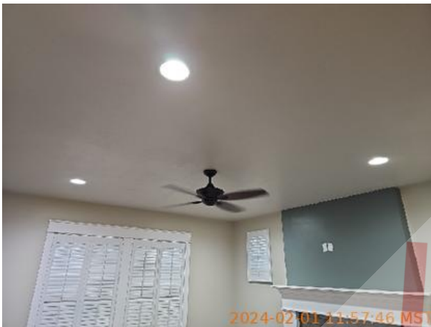
Light Fixture/Fan 📅 2024-02-01 11:57:46 📍 43.5756363, -116.1337315 🖼️ Image
