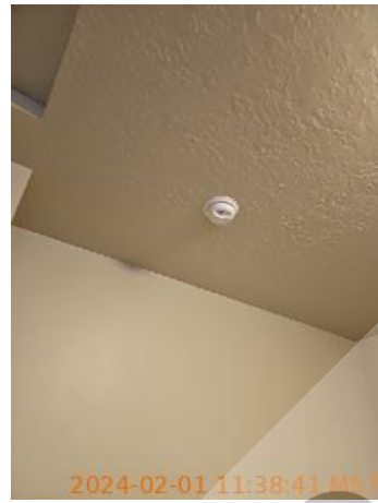
Smoke / CO detector
