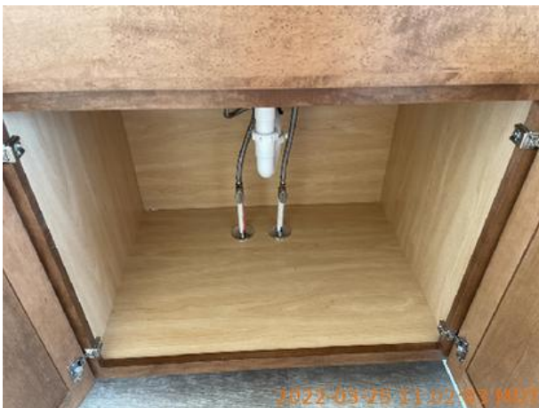
leak check 📅 2022-03-25 11:02:03 📍 43.72453506659097, -116.4868435284089 🖼️ Image
