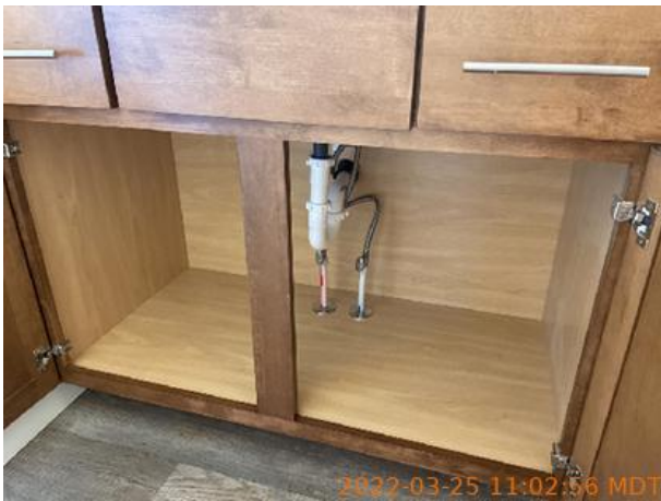
leak check 📅 2022-03-25 11:02:56 📍 43.72453506659097, -116.4868435284089 🖼️ Image
