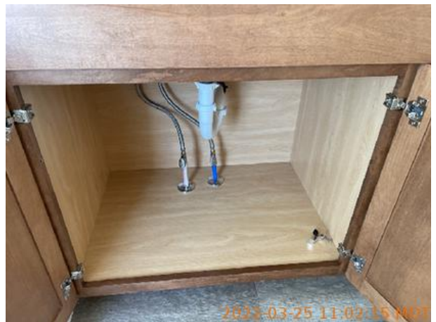
leak check 📅 2022-03-25 11:02:15 📍 43.72453506659097, -116.4868435284089 🖼️ Image
