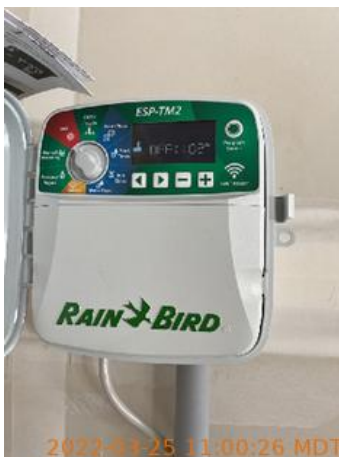
Sprinkler Timer Box
