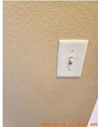
Switch/Outlet Taken on: 2019-01-30 11:18:50 Taken at: 43.70714458, -116.62559279 Image
