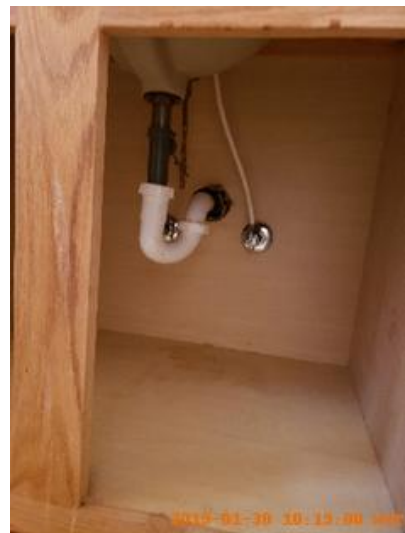
Plumbing/Drain Taken on: 2019-01-30 10:19:00 Taken at: 43.70723881, -116.62572328 Image
