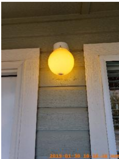
Light Fixture Taken on: 2019-01-30 10:16:16 Taken at: 43.70724052, -116.62561547 Image
