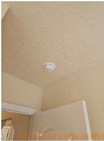
Smoke / CO detector
