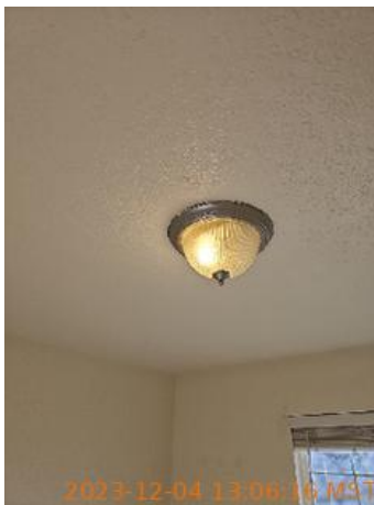
Light Fixture/Fan 📅 2023-12-04 13:06:16 📍 43.6959292, -116.4917973 🖼️ Image
