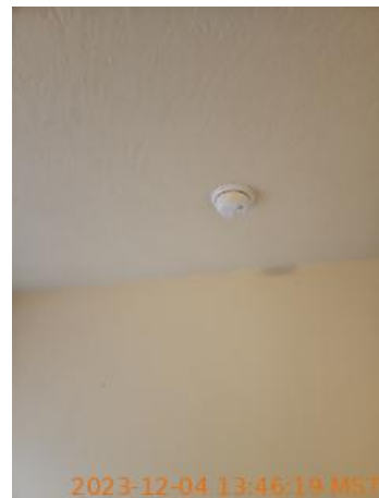
Smoke / CO detector
