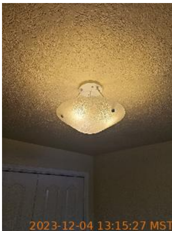
Light Fixture/Fan 📅 2023-12-04 13:15:27 🔍 43.6960637, -116.491778 🖼️ Image
