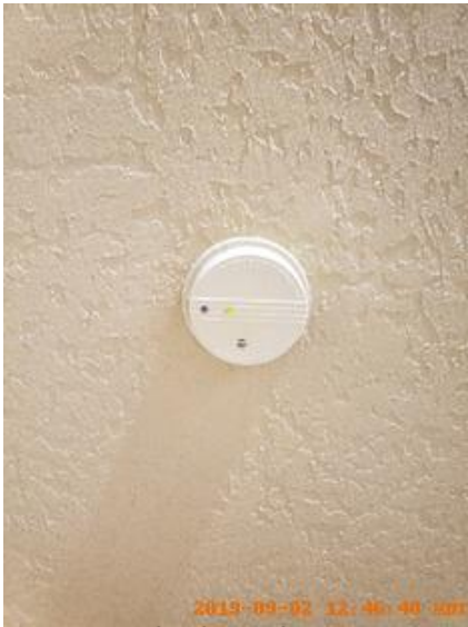
Smoke / CO detector
