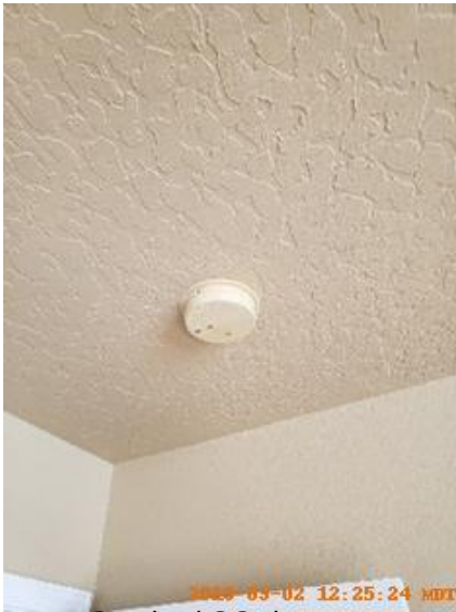
Smoke / CO detector
