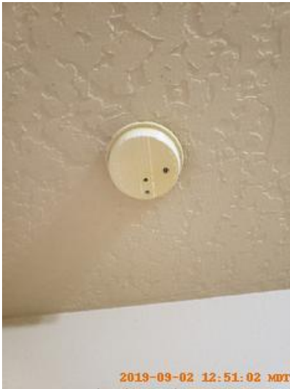
Smoke / CO detector
