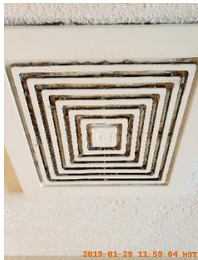
Exhaust Fan Taken on: 2019-01-29 11:59:04 Taken at: 43.56530939, -116.60391027 Image
