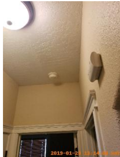
Smoke/CO Detector Taken on: 2019-01-29 13:14:08 Taken at: 43.56529839, -116.60395282 Image
